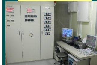
3. Monitoring & Management Room
